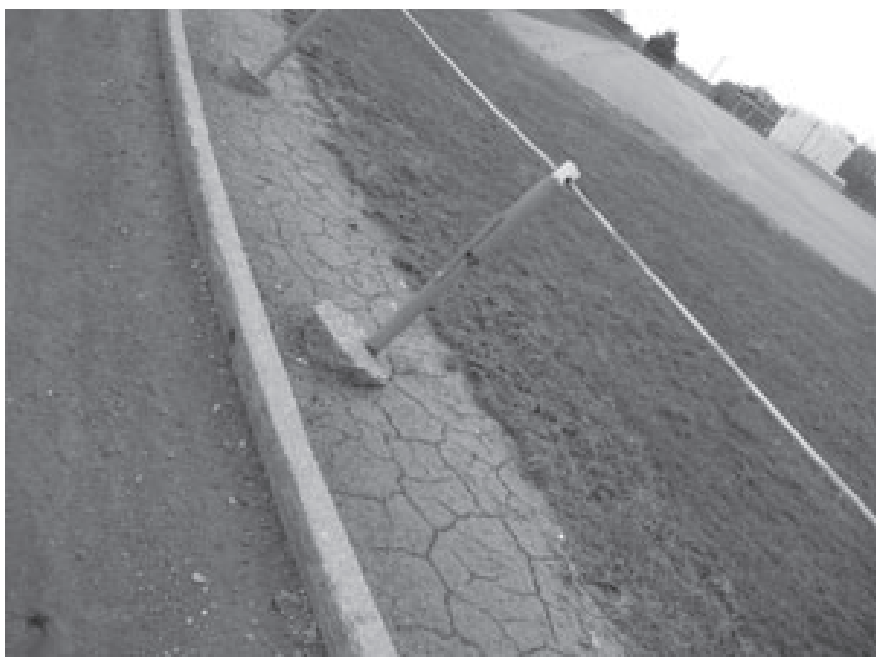
The old track is worn out
